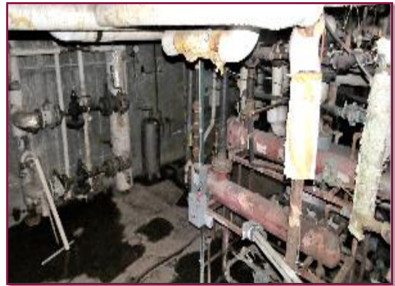
Aged Infrastructure Mechanical Room
