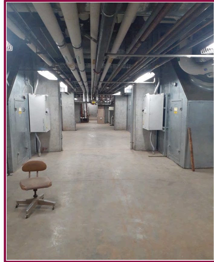
Air Handlers and Plumbing
