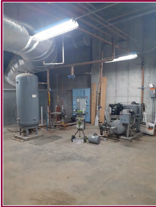
Compressor and Vacuum Pump
