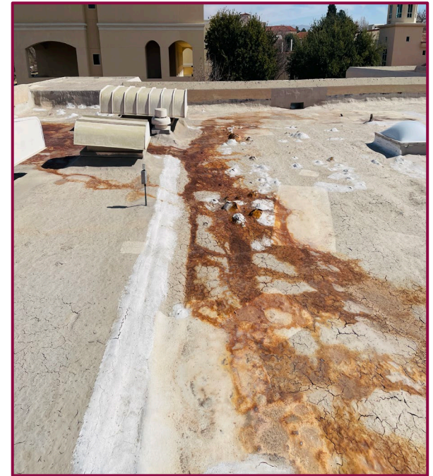
Dirt staining, cracking and bubbling of the roof
