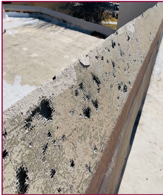
Parapet worn down with holes allowing water intrusion
