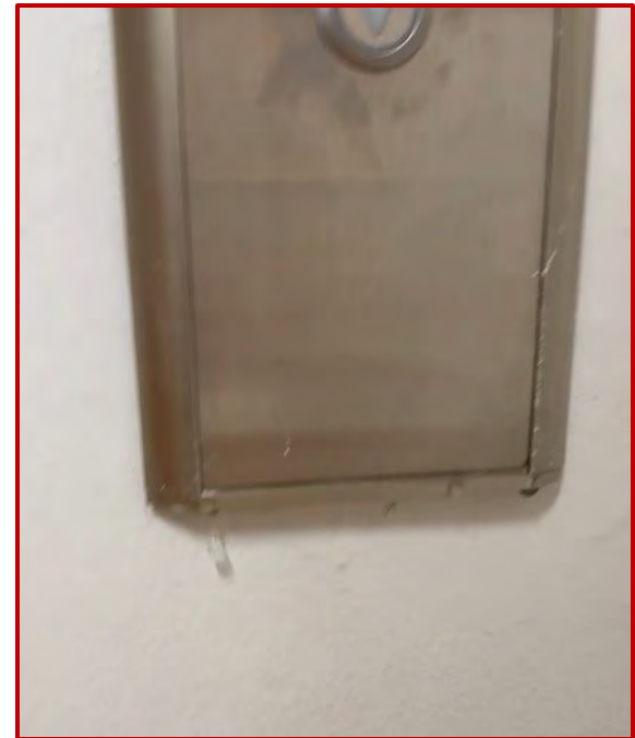
Water leaking from elevator button
