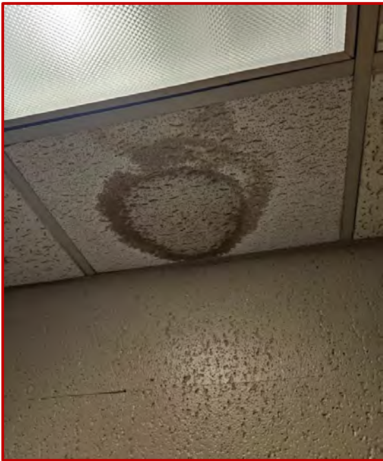
Water damage, room 201
