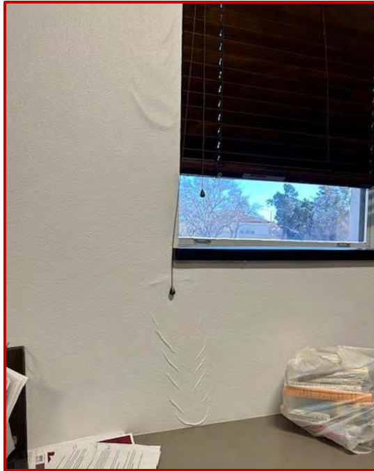
Water damage, room 125
